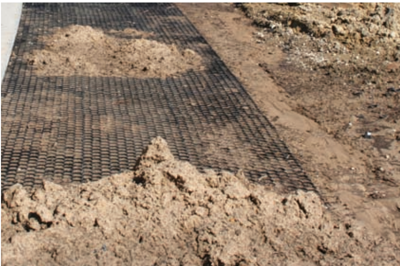
The Tufftrack was installed in 6 ft. wide strips, then backfilled with soil.
